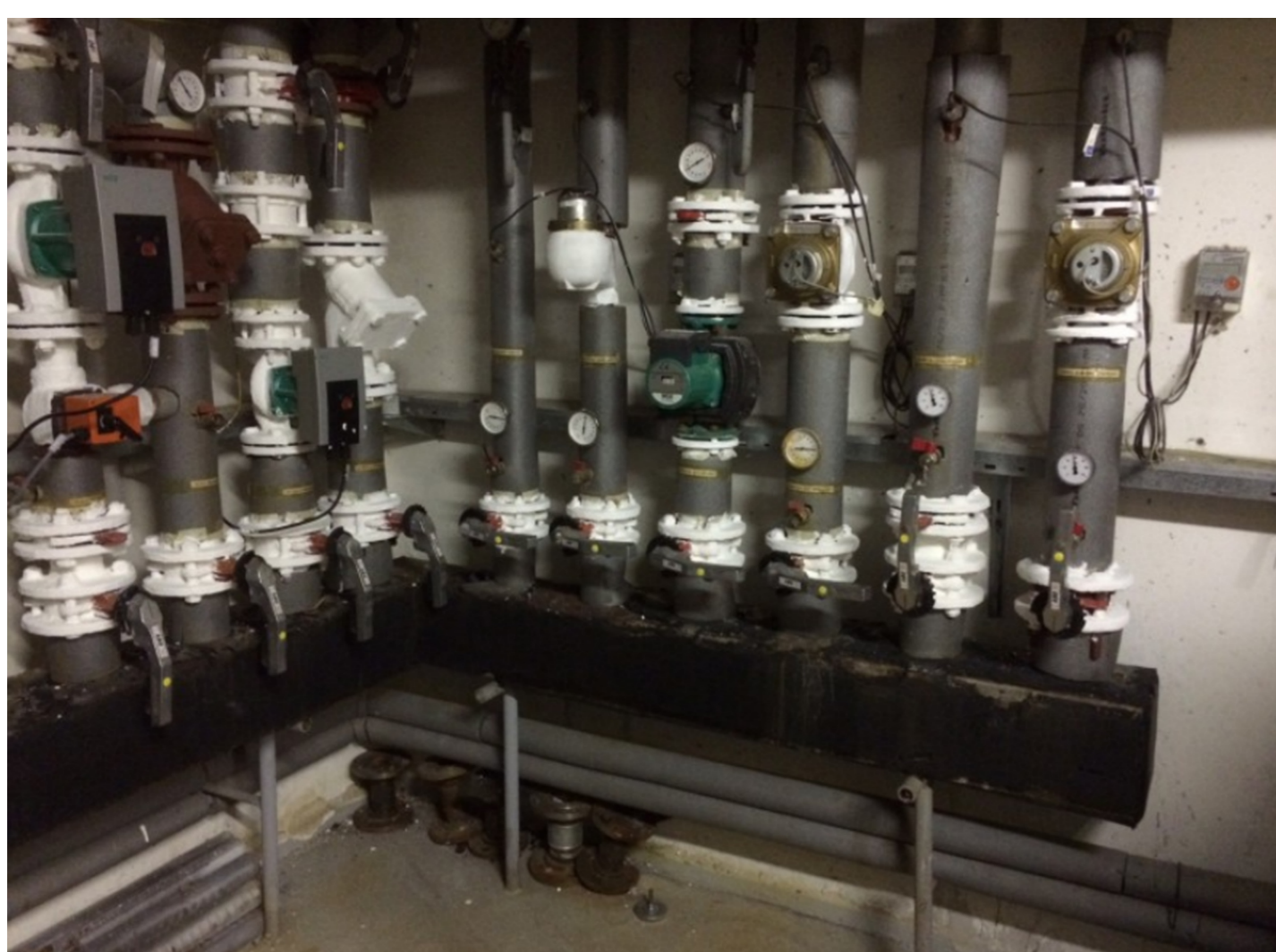
Additional insulation of fittings, Source: photo archive of the Aditex spol., s.r.o. company
