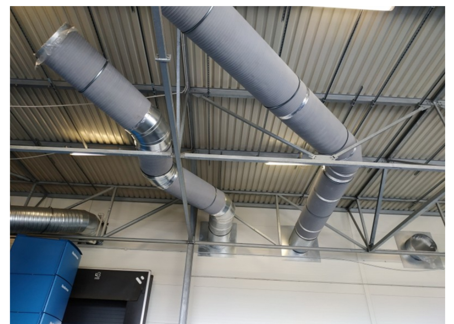
Insulated ductwork, Source: photo archive of the Aditex spol., s.r.o. company
