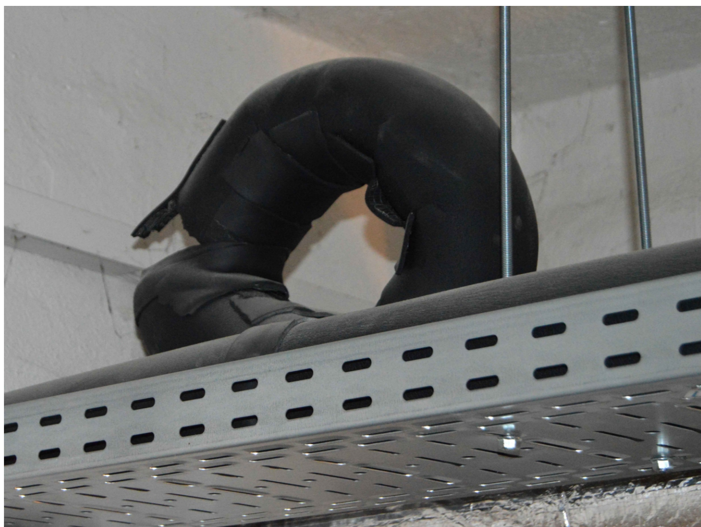
Problematic thermal insulation of more complex distribution routes, Source: author's photo archive
